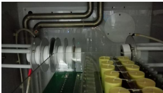
HV multiplier (front) with damaged capacitors and broken bleeding resistance (back)
