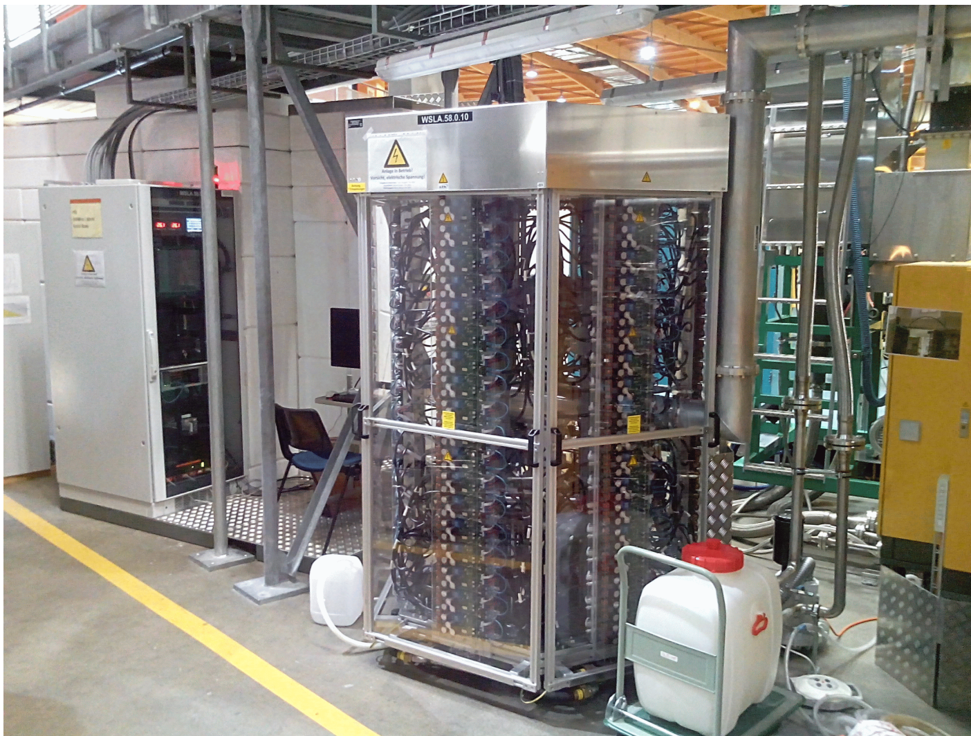
65kW 500MHz Solid-state Power Amplifier System Installed in SLS.
