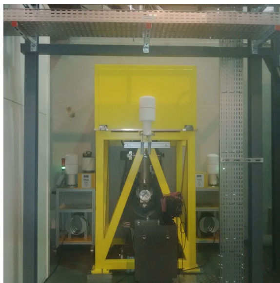
MIRAS shielding and radiation monitors.
